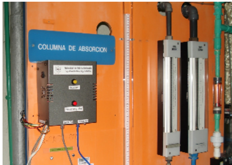
Figura No. 117 Panel de control instalado
