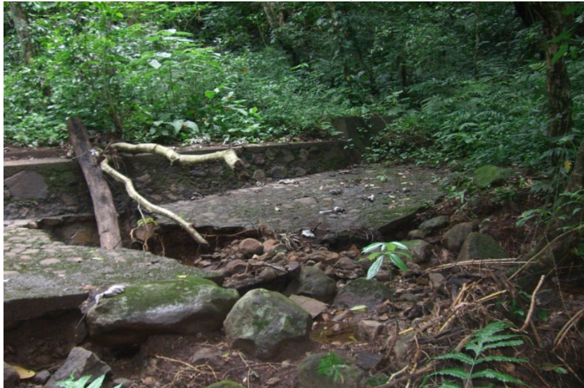
4.11 Manantial Santa Rita, losa dañada
