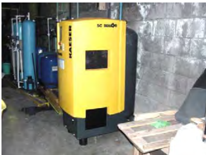
Figura 9: Compresor Airtower 5C
